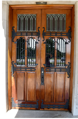
The front doors of the church have been restrained and sealed.
